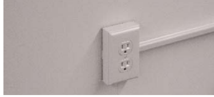
SURFACE WIRING CAN ALSO BE RUN HORIZONTAL IF THERE IS NO ELECTRICAL OUTLET IN THE JOIST/TRUSS CAVITY ASLL WILL BE INSTALLED IN.
