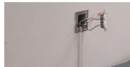
INSTALL SURFACE WIRING BOX PLATE ON EXISTING OUTLET AND WIRE POWER FEED IN FOR ASLL.
